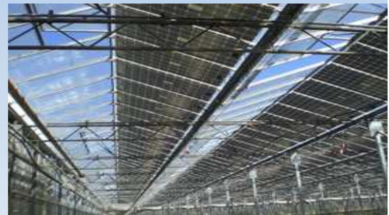
Montélimar , FRANCE 2.5 MW PV plant
